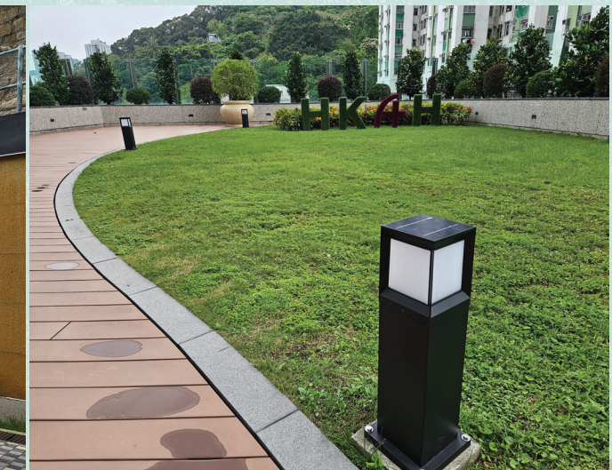
Solar-powered light poles installed at the 6/F sky garden and G/F parking areas 六樓空中花園及地面停車場安裝太陽能燈柱
